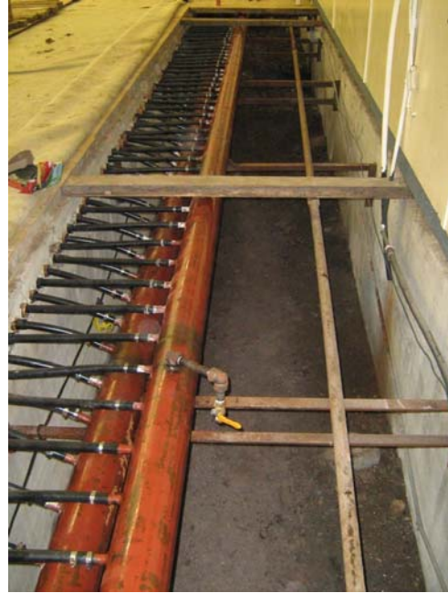
Header pipes After
