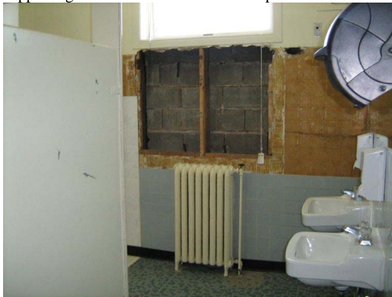
Wall under window in Men's washroom
